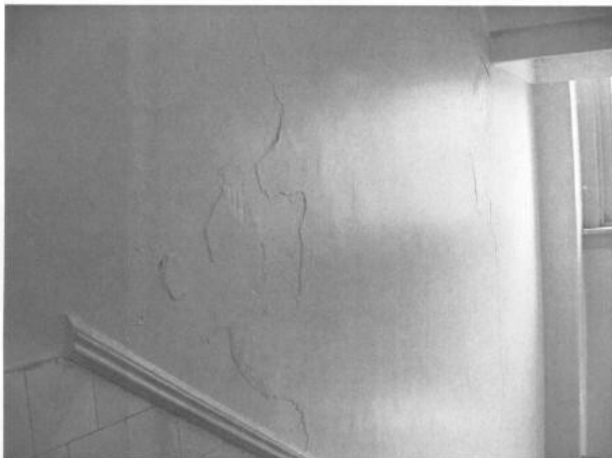
PS 138 Brooklyn, Photograph #8, Inadequate Plaster Patch and Repair Work at Stairway
