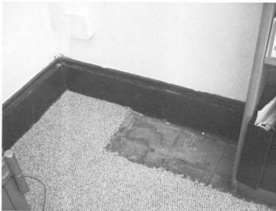
IS 228 Brooklyn, Photograph #4, Missing Carpet and Vinyl Base in Principal's Office
