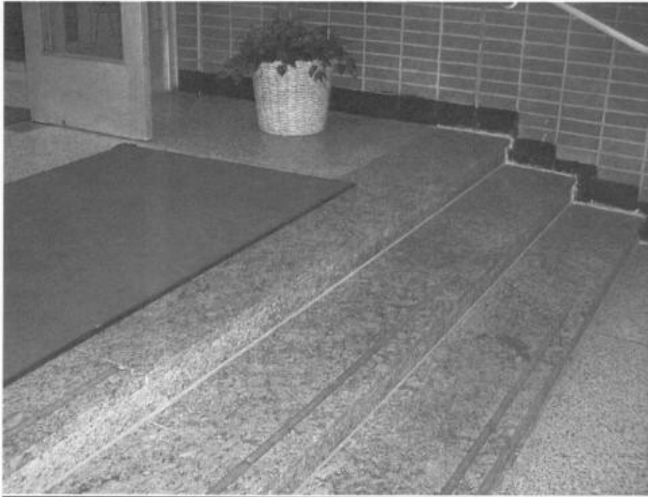
PS 262 Brooklyn, Photograph #5, Missing Adhesive Strip in Lobby Steps
